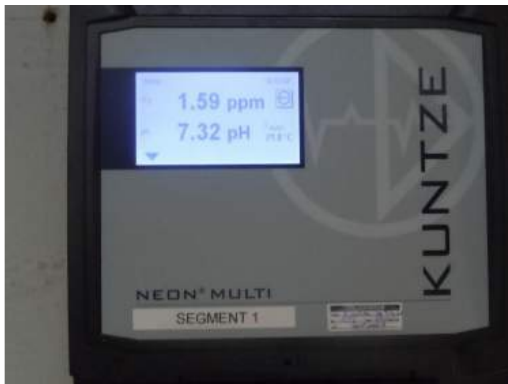
Photo 2-6: View of On-Line pH & Free Cl Residual Monitoring Analyzer
